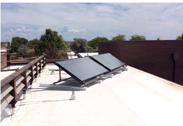
Loven Contracting installed a roof-mounted photovoltaic array and tied it into the existing power system.
