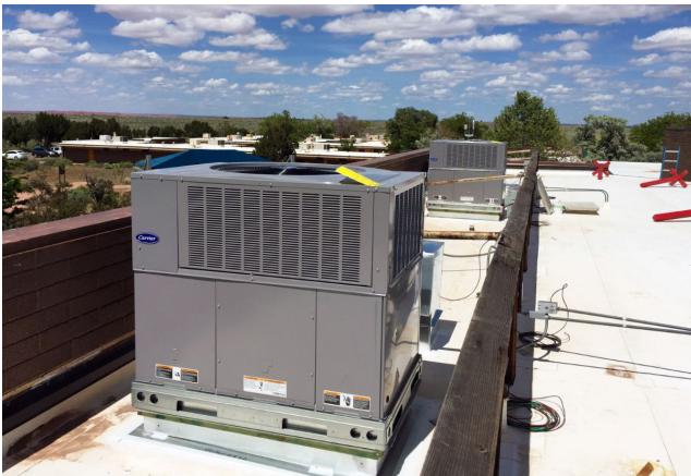
The existing air conditioning units were replaced with more efficient models able to better serve the Community Building.
