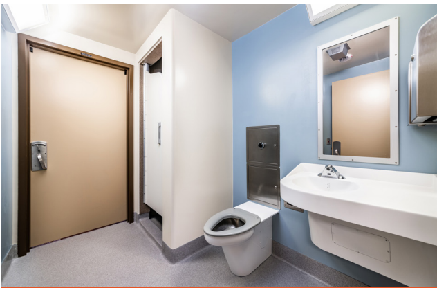
The restrooms are equipped with tamper-proof features, including anti-ligature shower doors, solid surface shower surrounds, and epoxy flooring.
