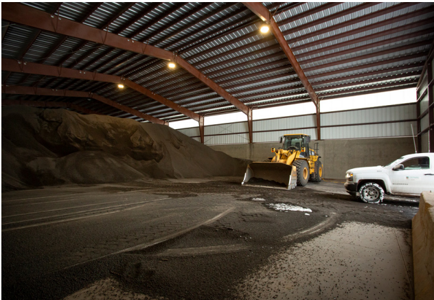
Concrete slab thickness was calculated to meet both budget requirements and long-term durability issues relative to the equipment and cinders' weight.
