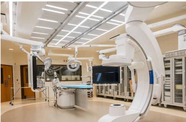
The new operating room is lead shielded, equipped with an upgraded air flow and med gas with ultrasound equipment and new finishes.
